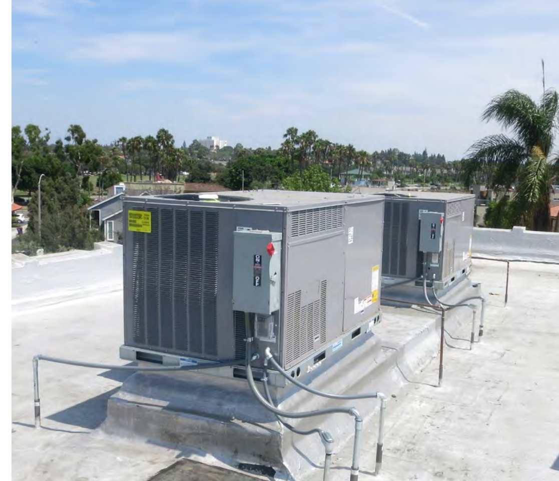
5 ton rooftop heat pump.
